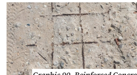
Graphic 90- Reinforced Concrete Durable, affordable and with a high load capacity. Can be used for bearing walls or paths.
