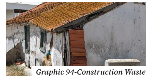
Graphic 94-Construction Waste Leftover bricks or beams can creatively be used to stabilise existing structures.
