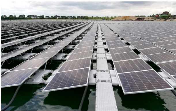
Figure 8: Tilted air cooled panels on plastic floats from SunEvo Solar. Source: SunEvo Solar [17].
