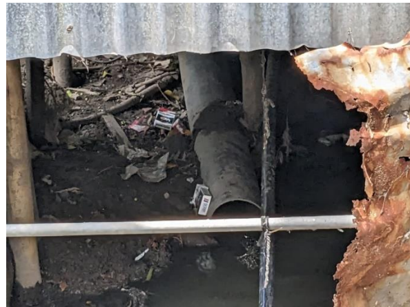
Fig. 55: Water still persists under ground of such a house.
