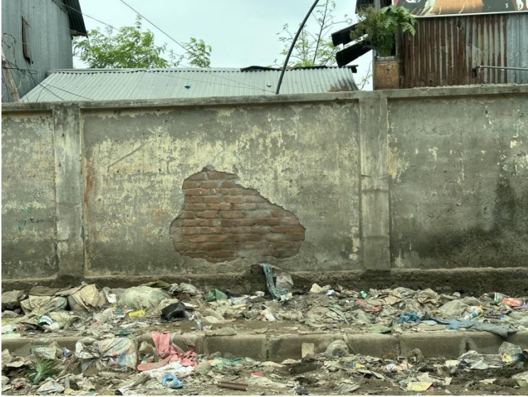
Fig. 44: Dumping of Waste in Nearby Roads.
