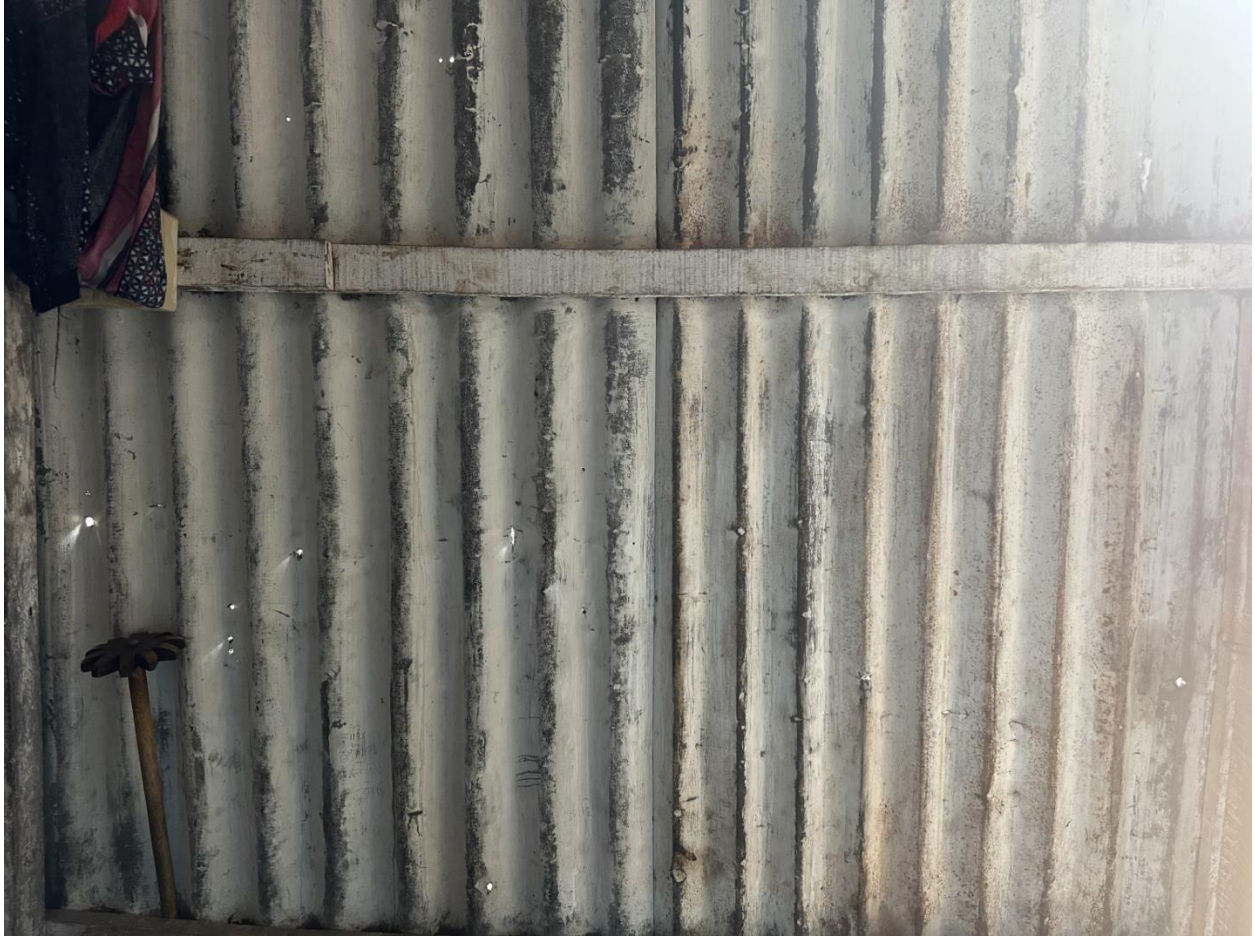
Fig. 59: Tin sheet with holes are used as readily available material to build houses.
