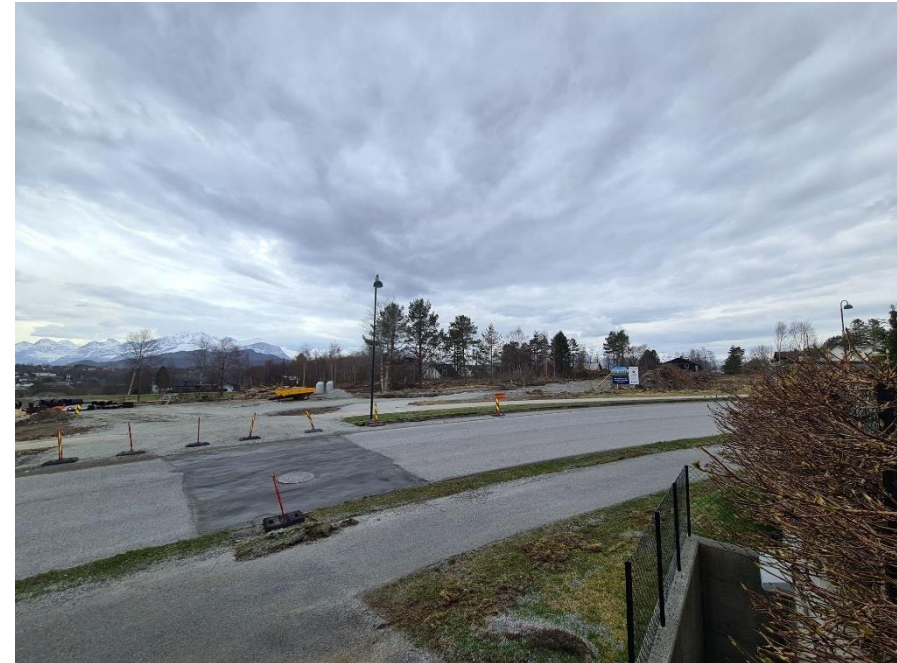
Figure 37: How the building site looks today. The existing forest was completely cut down and removed to prepare the area for construction.
