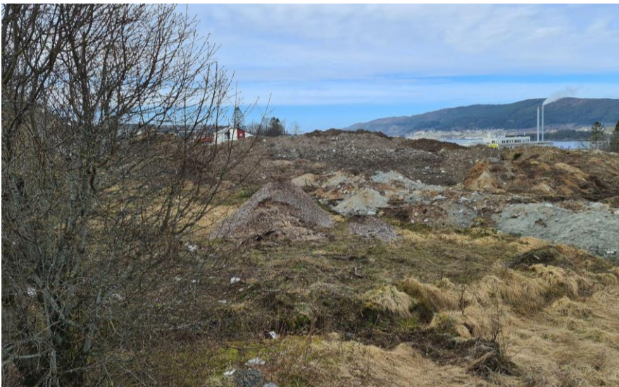
Figure 43: Removal of the natural substrate to make space for the utility's necessities for households.
