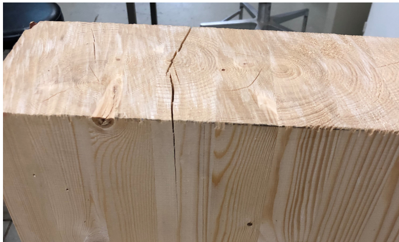
Figure 6.14: Defects in timber
