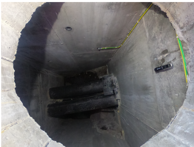
(a) View of the manhole and the LASCAR EL-USB-2 Temperature USB Data Logger placement.
