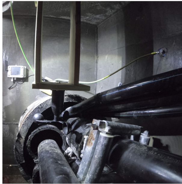
(a) The mounting bracket and placement of the UBIBOT wind sensor and the UBIBOT GS1-AL4G1RS Industrial Logger at the outlet basin.
