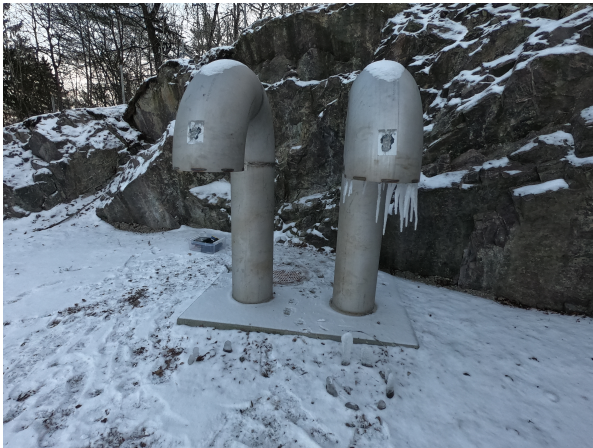
(b) Outside of the outlet basin where the two ventilation goose neck pipes are fitted.
