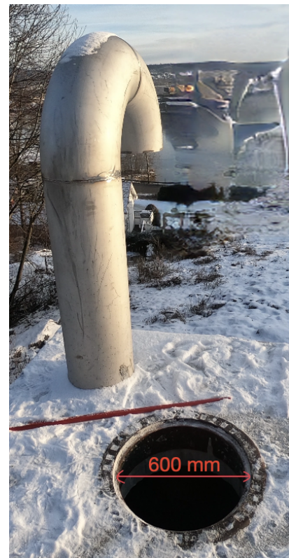
(b) Outside of the inlet basin with goose neck ventilation inlet and manhole for accessing the logger. The manhole is 600 mm wide.
