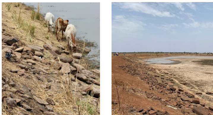
Figure 6. Rip rap lining of the dugout wall as a measure to avoid soil erosion.
