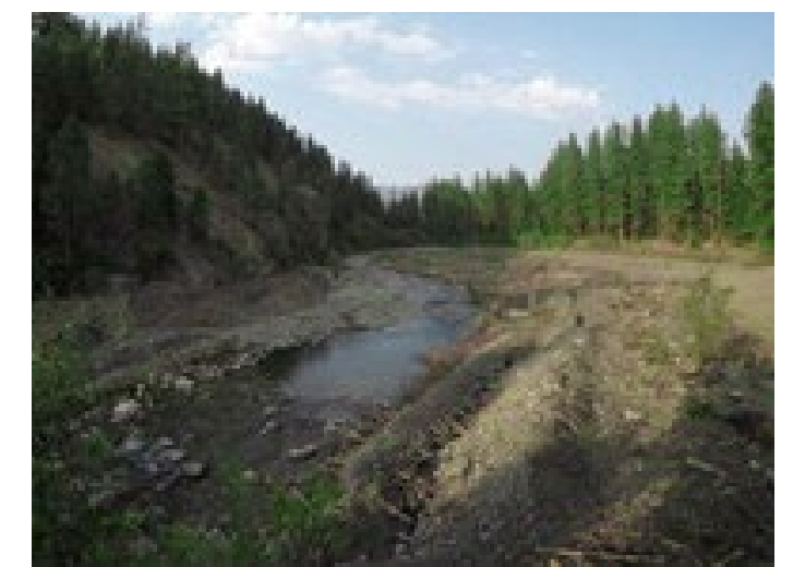
Figure 16e: Former Dam Site Ready for Revegetation (Image source: City of Missoula, no date).
