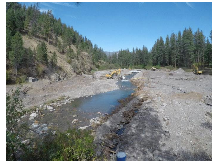
Figure 16d: Creek Excavation Starting to Wrap up (Image source: City of Missoula, no date).
