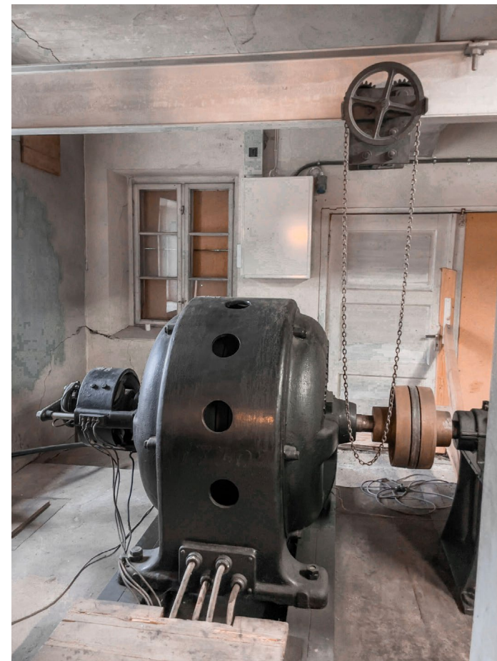
Figure 44c: Generator unit (Photo: Fjeldberg, I. 2022).
