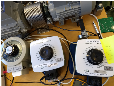
Fig. 49. The three autotransformers. Note that the connection to the left on each autotrafo designates the ground on the secondary side, are all connected together. The motor in the background are not relevant for the demonstration.
