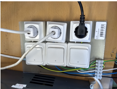
Fig. 50. A basic, but practical connection board connecting the secondary side of the isolation-transformer with the autotransformers
