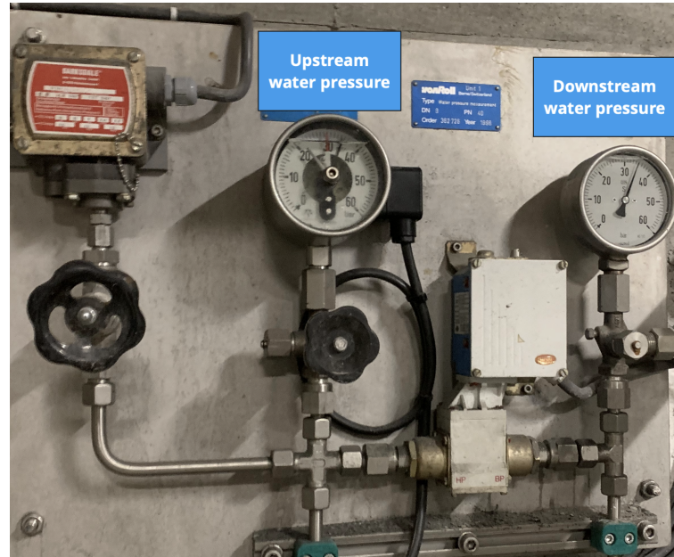
FIGURE 3.2: Pressure measurements downstream and upstream of valve 1 at Nore 1 HPP.
