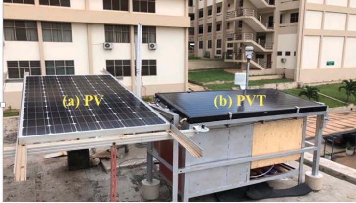
Fig. 1. PV (a) and PVT (b) installation on the rooftop of Solar Energy Applications Laboratory at Department of Mechanical Engineering, KNUST Ghana [26].
