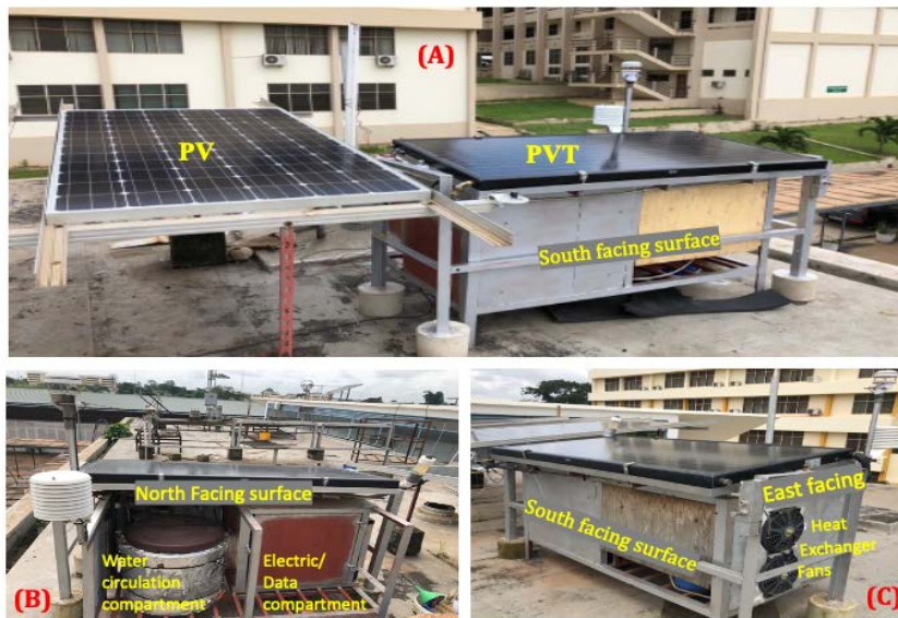
Figure 3.10: Installation of setup on the roof top of Solar Energy Applications Laboratory at Department of Mechanical Engineering, KNUST Ghana, showing: (A) PV and PVT modules; (B) North facing surface with water circulation and Electric/Data compartments; (C) East facing surface with radiator cooling fans
