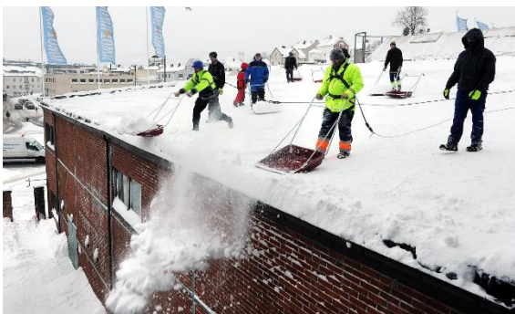
Figure 9. Snow load control at Down Town shopping center before installing PV heating system, manually shoveling the snow. (FUSen, 2021)
