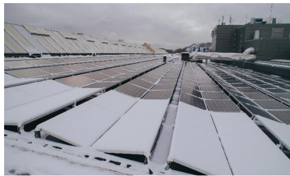
Figure 8. PV heating system installed at Down Town shopping center. A total of 6000 m 2 of PV panels with heating systems for melting are installed on the flat roof. (FUSen, 2021)
