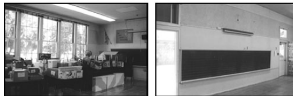
Photos of Daylight Code 4 Classrooms North Windows (left) and South Windows (right)
