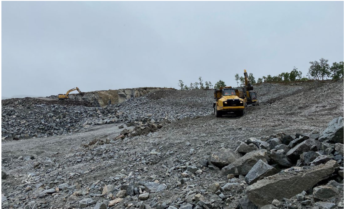
Figure 2.1.5-2: Stone quarry for hydroelectric power dam rehabilitation approx. 960 m.a.s.l., Songa dam, Vinje municipality, Vestfold and Telemark County. Photo: Line Rosef
