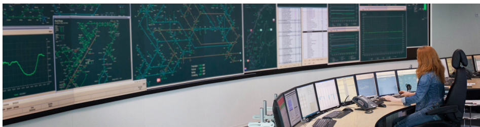
Figure 5.1: The national central office ( Landssentralen ) at Statnett [45].
