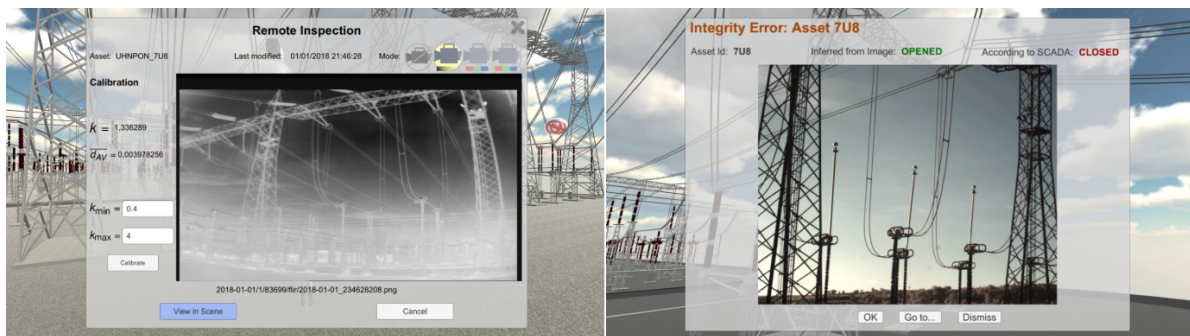
Figure 7.6: Remote inspection of a substation. Camera options and metadata are provided [80]. Courtesy of Leandro Mattioli.
