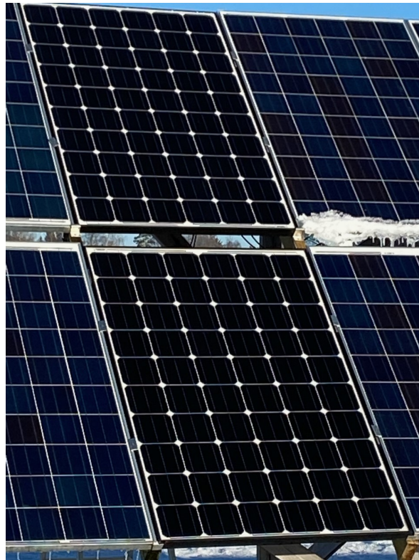
Figure 2.2.1: Image of PV-cells (the small black squares) in a PV-module connected in a PV-array.
