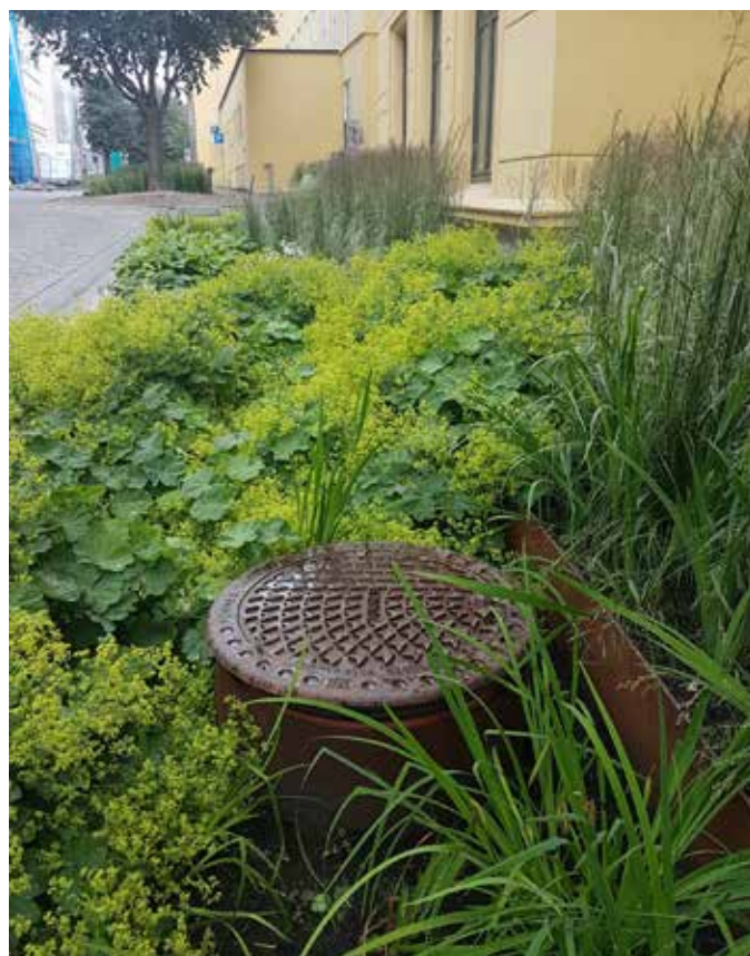
Photo 6.3 Infrastructure in the rain garden
