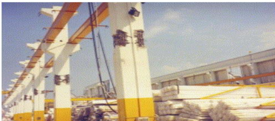
Figure 2-10 it shows by the lack procedural structural design the failure of column (Arslan, 2006)
