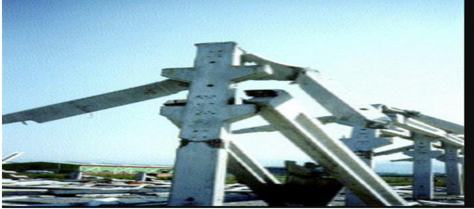
Figure 2-13 it shows the damage of precast reinforced concrete during earthquake in most building in Turkey (Arslan.et.al,2006).
