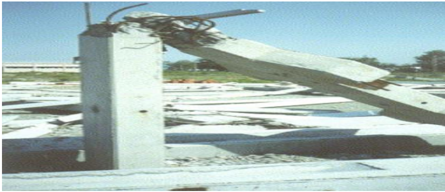
Figure2-12 it shows the damage of joints of precast during earthquake (Arslan.et.al,2006)
