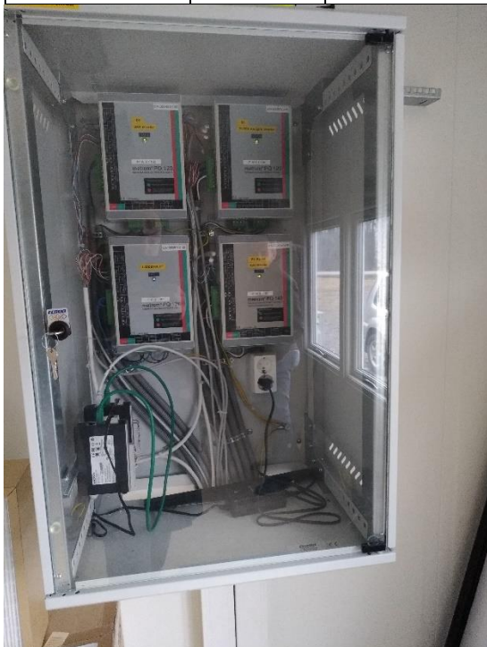
Figure 4: The four inverters at for the different plants at GEC. Photo: Jesper Frausig.
