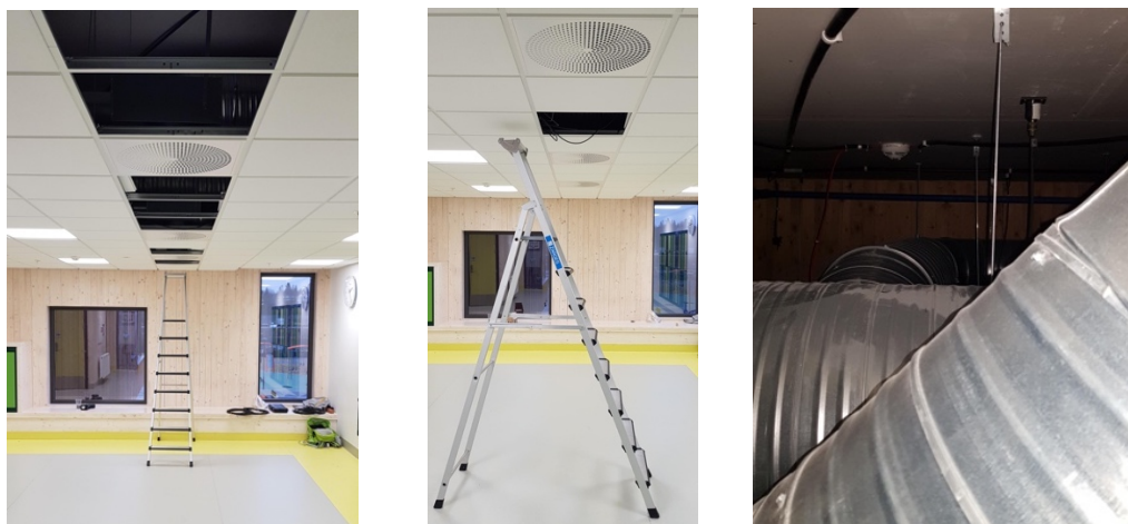
Figur 29: Oppkobling over systemhimling (privat).
