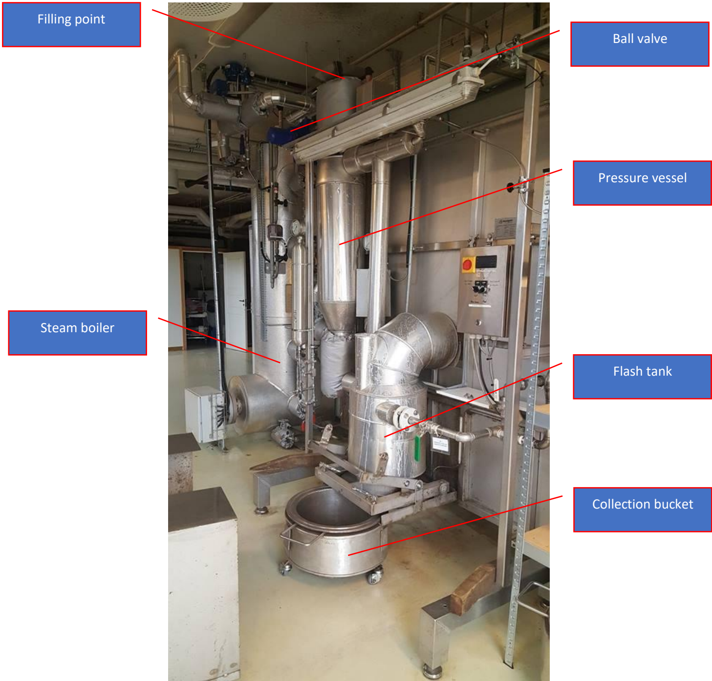
Figure 2.4: Picture of the steam explosion unit with markers to show the main parts.
