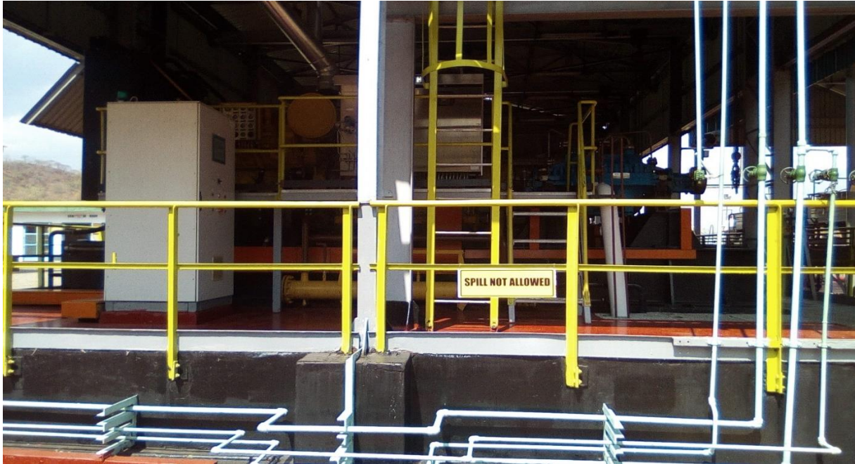
Picture 5: Kisanga pumping station, one of the pumping stations along TAZAMA pipeline route (Photo by author)
