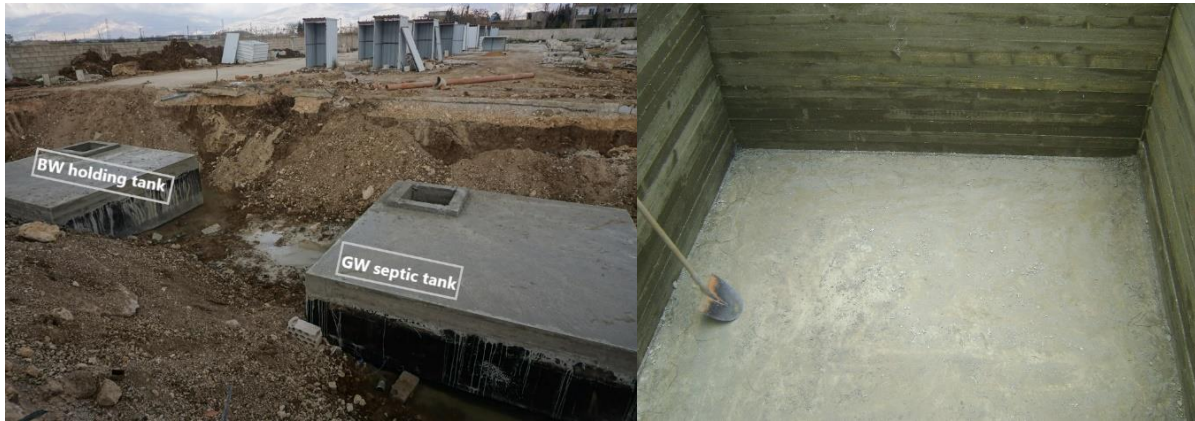
Figure 5.1 (left): The BW holding tank and GW septic tank in Yasmine camp (Photo: NCA, 2016), Figure 5.1 (right): Inside the one-chamber BW holding tank (Photo: IOCC, 2014)
