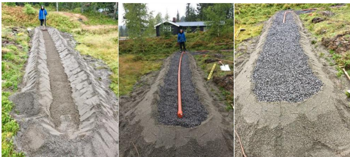
Figure 5.6: Construction of a mound system for a small cabin in Norway (Photos: Petter D. Jenssen)
