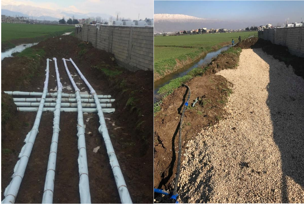
Figure 4.3 (left): The way the pipes cross each other in the soil infiltration trench in Awda camp, Figure 4.3 (right): Backfilling with a layer of gravel over the natural underlying soil and pipes
