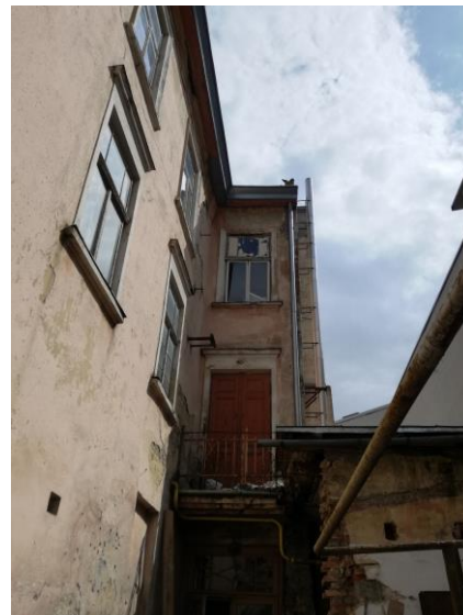
Figure 2-37: Courtyard. Remaining balcony after the dismantled stairs. (Author, 2018).
