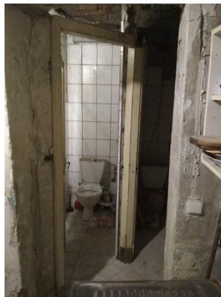
Figure 2-33: Toilets. Toilet units. (Nazar, 2018).
