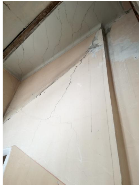
Figure C26: Staircase. Cracks on the walls and ceiling. (Author, 2018).
