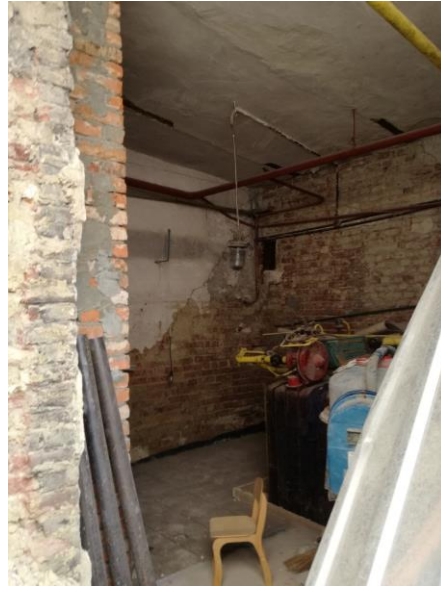
Figure C6: Boiler room. (Author, 2018).
