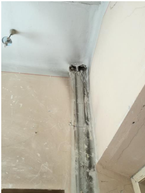
Figure C25: Staircase. Burn marks after old heating pipe system. (Author, 2018).
