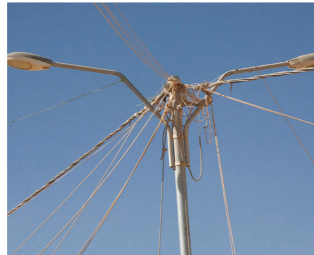
The total number of kilometers with illegal electrical wires in the refugee camp are: 300 km (Ledwith, 2014).
