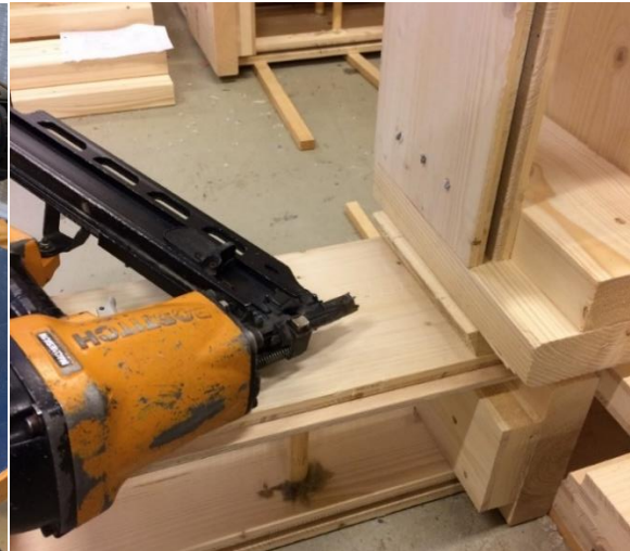
Figure 3-11: Attaching Termowood element to middle sill with a 60-degree angled nail connector.
