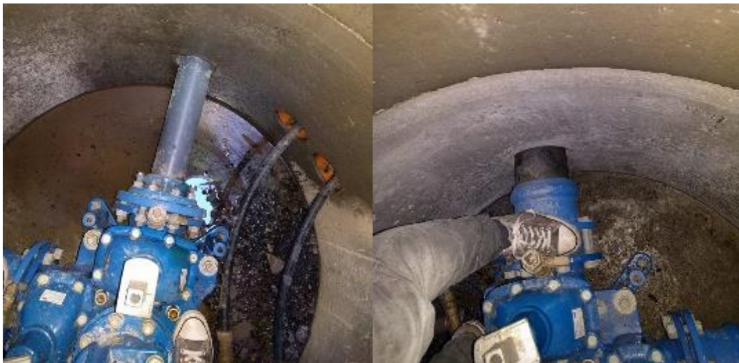
Figure 24: Inspection of second manhole revealed multiple places a clamp-on flow meter could be installed (Photo: Kevin Vesterås).
