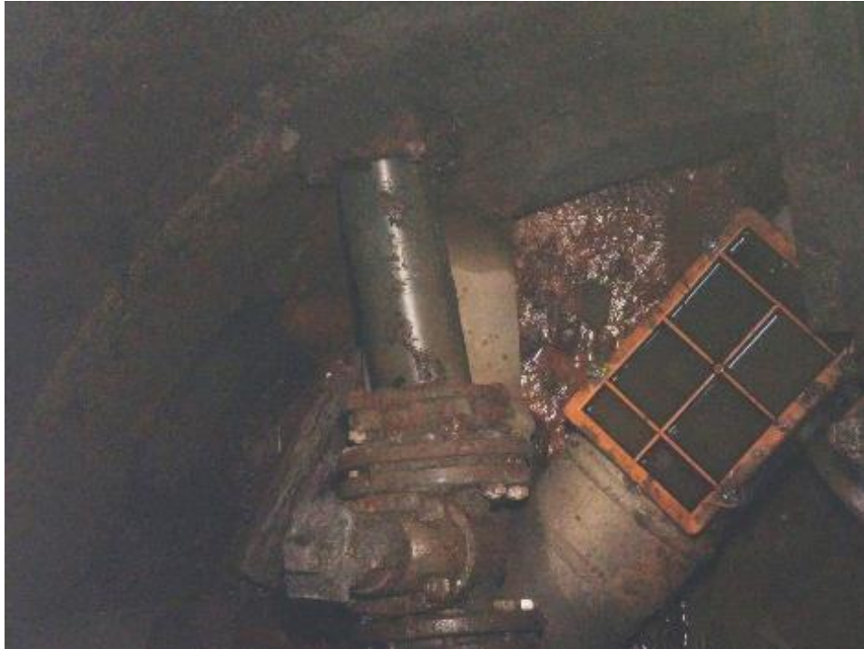
Figure 23: Inspection of the first manhole revealed a suitable placement of a flow meter, although in a dirty environment (Photo: Kevin Vesterås).
