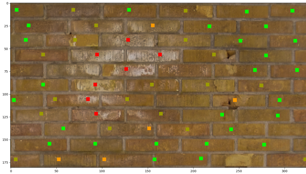
Figure 6.3: Here we see the prominence of white salt on the bricks. This texture causes the entropy value to be high and it is therefore categorized as red. Even though the structure of the bricks are good in this area. This area is located on the right side of the East wall.
