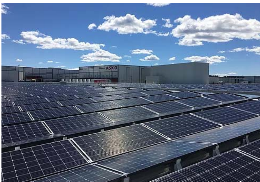
Figure 5-4 Solar PV at ASKO, Vestby. Source: Fusen.no
