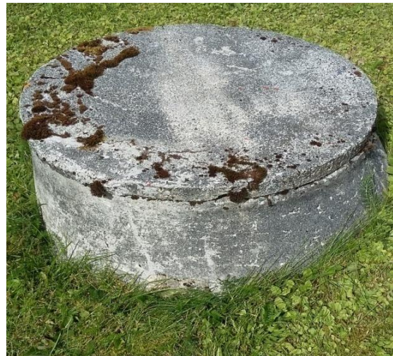
Figure 3: Cement based septic tank with the volume of 2m 3 and 1 chamber
