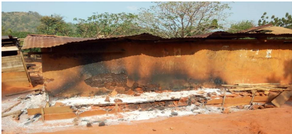
Figure 6 A house burnt down by herders at Hweehwee area
