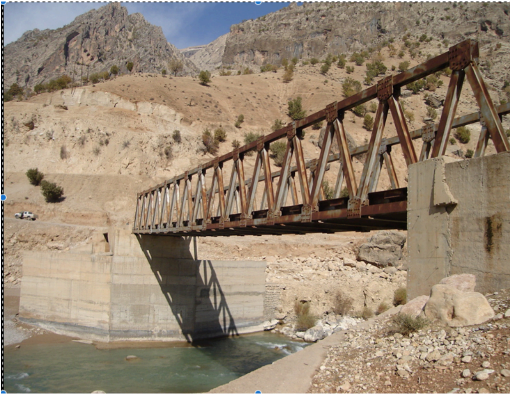
Figure 1- Talaeih metal bridge which was located on the upstream of dam site.
