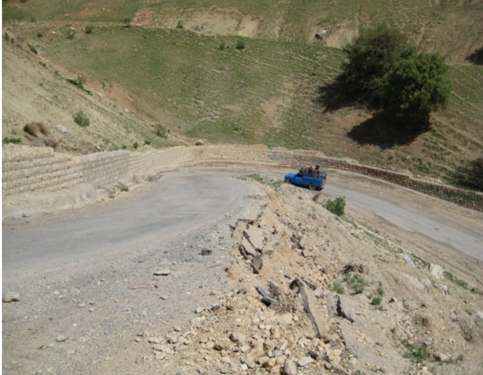
Figure 2- Inappropriate quality of the road in 4.80 Km after the Sardasht police station to the dam site.
