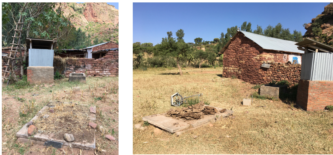
Image 3: Biogas installations in disuse. Note the photo on the right; manure is being dried on top of the digester.
