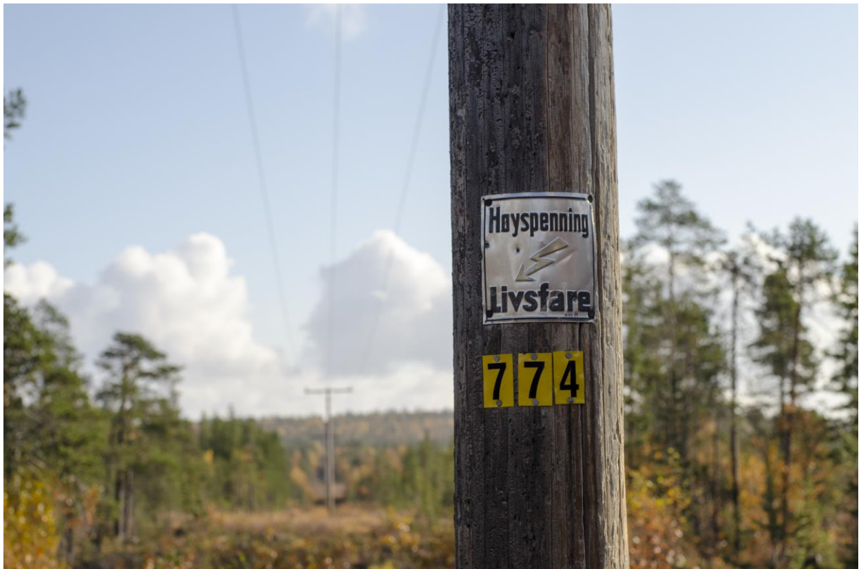
Fig. 1: Power pole in the Pasvik Valley, Norway. Every pole is registered by its unique number. Photo: Alexander Kopatz.
