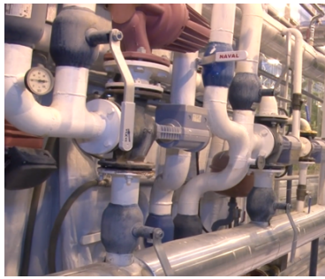
(a) Valves as part of the heat regulator of the greenhouse.
