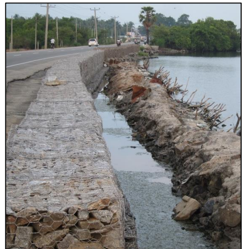
Figure 12 Gabions protecting the A15 highway from shore erosion in Sathurukondan.
