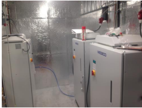
Figure 3.8.1: Wedeco Ozone generators (Levik, K., 2017b)
