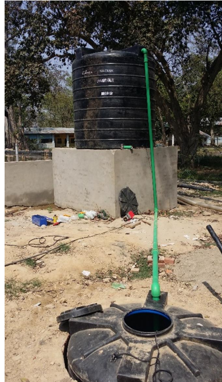
Figure 3: Pump tank (nearest) with piping to the biofilter (Photo: Anders Rørå).
