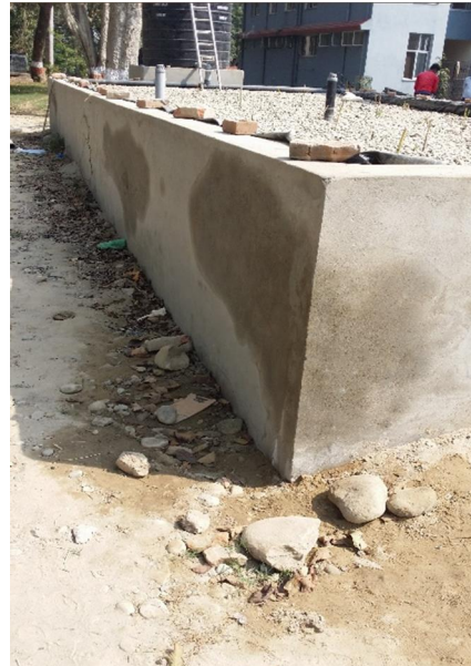
Figure 17: Wet spots on the wall and moist ground indicates leaking from the bed (Photo: Anders Rørå).
