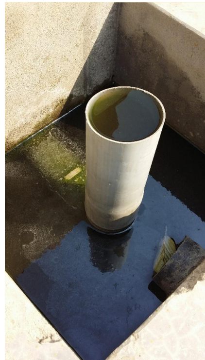
Figure 18: Outlet basin filled with water. The outlet is currently raised to allow the plants to form deeper roots (Photo: Anders Rørå).
