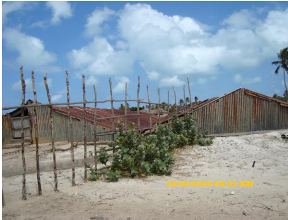
Figure 15: Rainwater harvesting infrastructure at Jibondo
