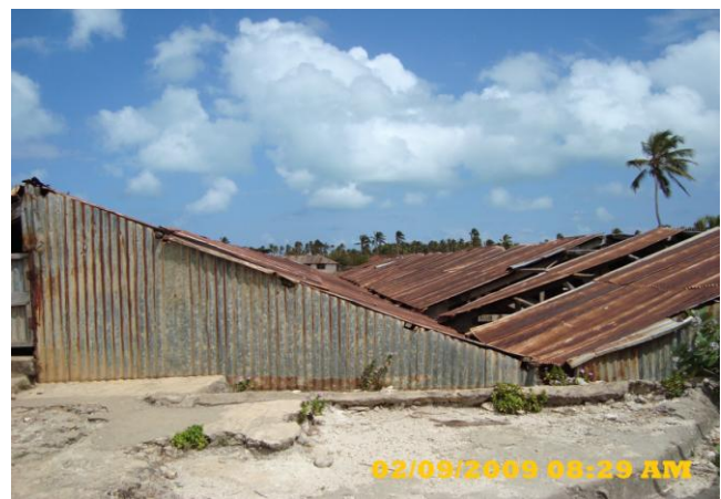
Figure 16: Worn out infrastructure at Jibondo that produce rusted water, unsuitable for human consumption
