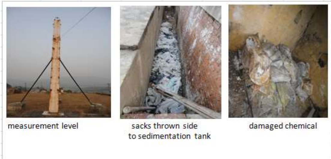
Figure 20: Observation at Bansabari Treatment Plant
