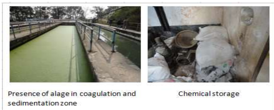
Figure 23: Field observation at Balaju Treatment plant
