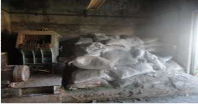
Figure 19: Condition of chemical storage facility at Mahankalchaur WTP
