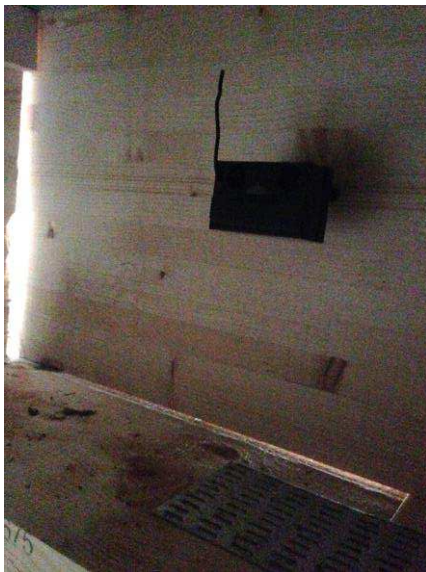
Figure 15: The placement of one of the sensors in the southern facing bedroom, where leaks between the joists are observed
