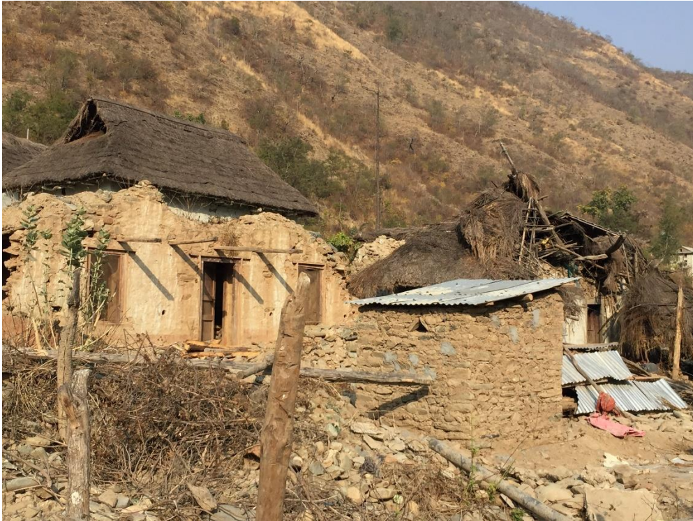
A broken house- Picture of broken house in Bhirpani taken by Neeraj Katwal during field visit on February 2016
