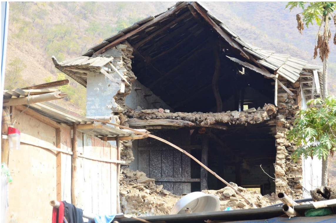
Another destroyed house in Rakathum
