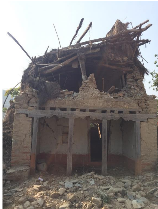
Photo: State of house in Rakathum destroyed by earthquake in April 2015 (photo taken in February 2016 during field visit)
