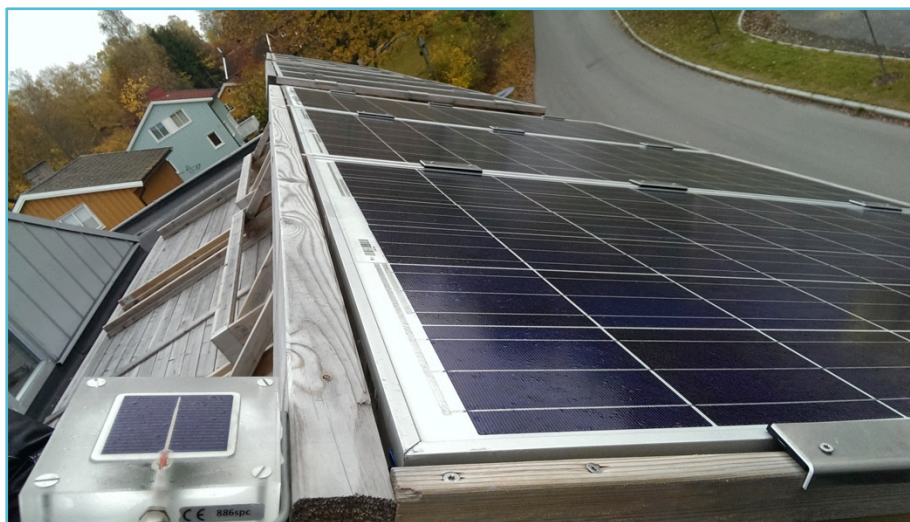
Figure 37: Photo towards the east of the PV-array at Aas
