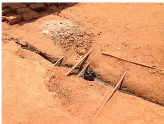
Drinking water pipes in the open with garbage around
