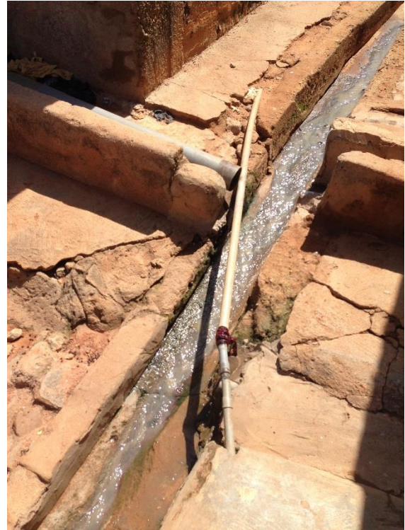
The leaking pipe is crosses above the grey water in the gutter
