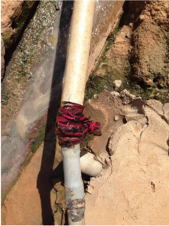
Leakage from a water pipe
