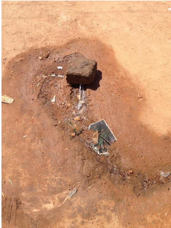
Hole in the water pipe exposed
