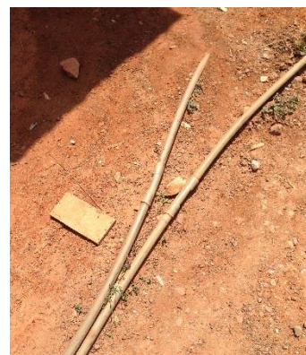
Drinking water pipes in the open
