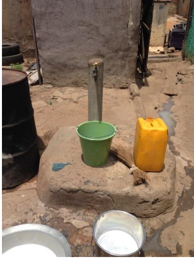
Typical water tap in the slum area
