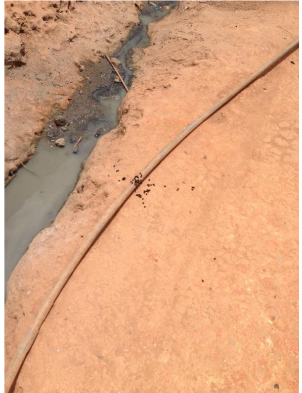
Animal feces on the drinking water pipe
