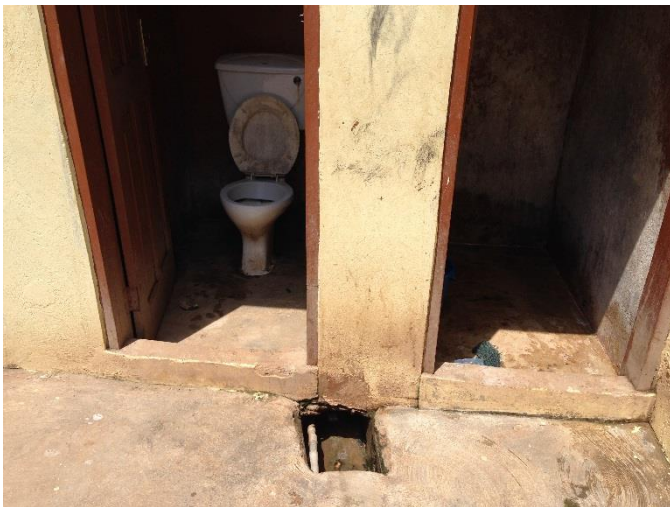
The water pipe is exposed and goes under the toilet and shower
