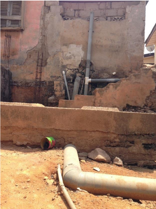
Many pipes laying close to each other. The drinking water pipes also goes trough the septic tank
