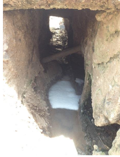
Drinking water pipe going through the gutter
