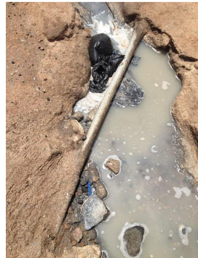
Drinking water pipe lying in the gutter together with grey water
