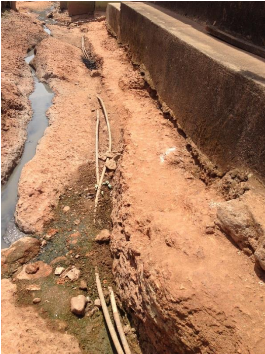
Exposed pipe going through the gutter
