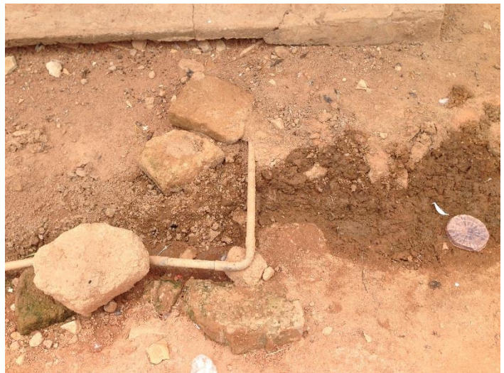
Stones are used hold the pipes stable and to take the pressure from the water
