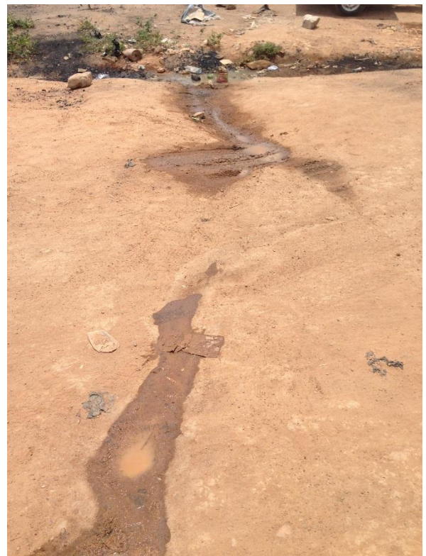
This picture is taken few days after the pictures above. Soil has been put on the top of the pipe ,but the hole is not fixed and water i leaking out in to the area
