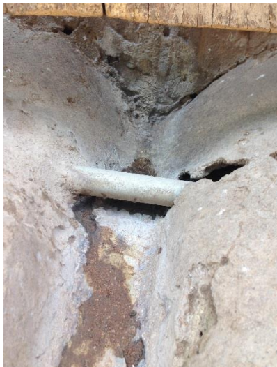
Drinking water pipe at the entrance in the door entrance
