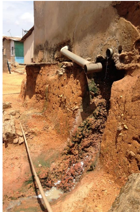
Drinking water pipe exposed to grey water
