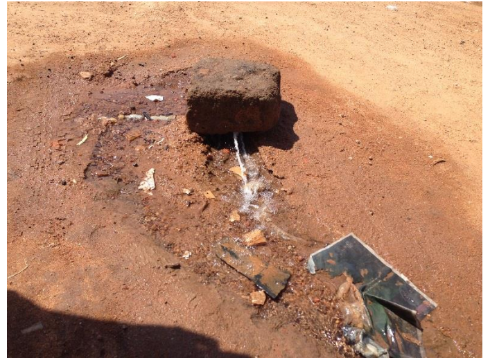
Hole in the water pipe
