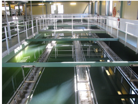
Figure 7.1 Sedimentation tank at the Drøbak WWTP, Norway
