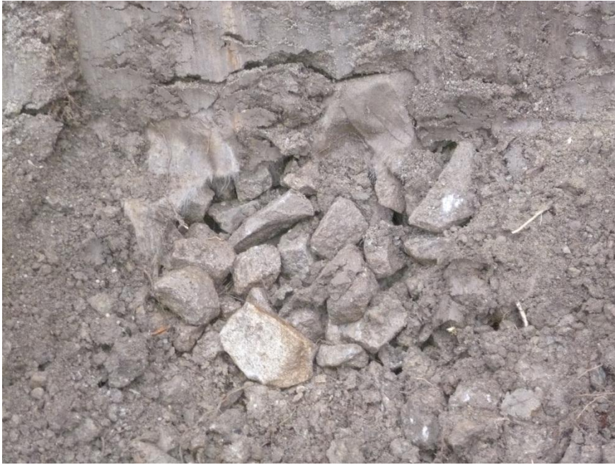
Figure 6. Large rocks and geotextile found in the bottom of the stop butt. (Photo: Liland, 2012)
