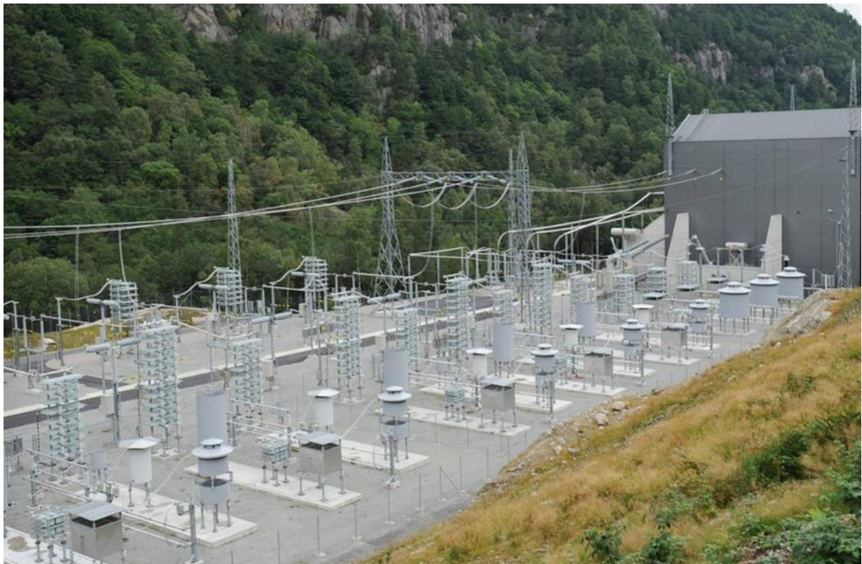
Figure 67: Feda station, onshore substation for the NorNed subsea power cable system (Tubaas & Olsen 2011)
