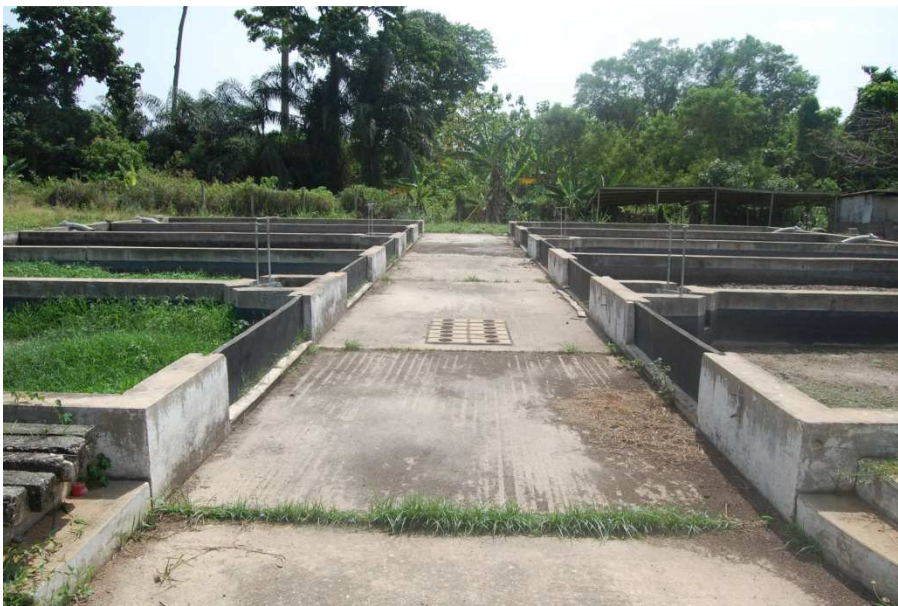
Figure 16: Sludge drying beds
