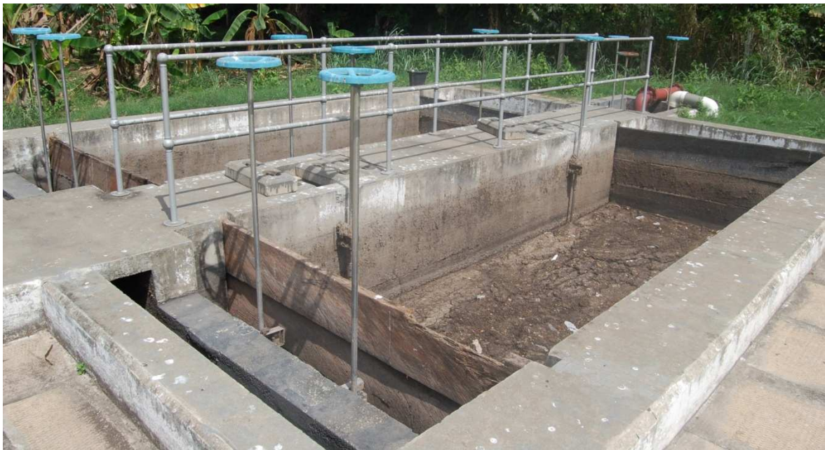
Figure 6: Primary sedimentation tank
