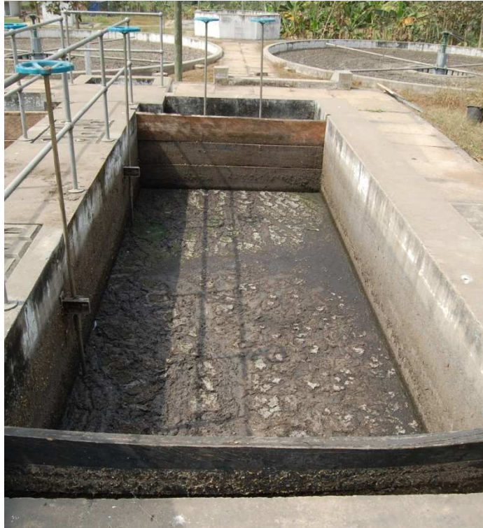
Figure 7: Primary sedimentation tank
