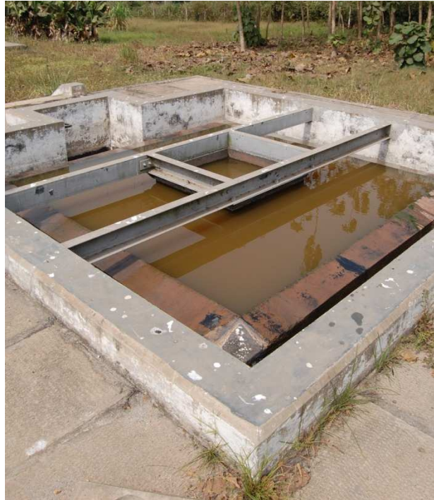
Figure 12: Secondary sedimentation tank
