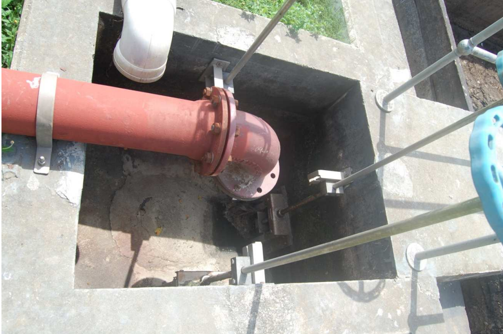
Figure 5: Inlet of primary sedimentation tank
