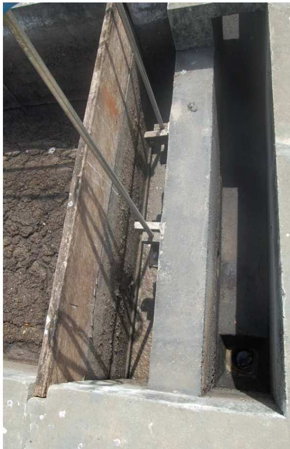
Figure 8: Outlet of primary sedimentation tank
