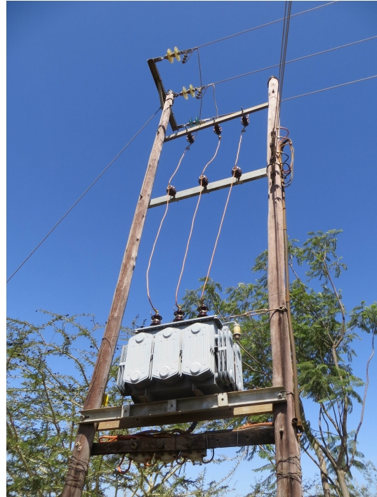
Figure 2.7: The 200 kVa, 11 kV/400 V transformer, connecting MCF Yatta to the grid.
