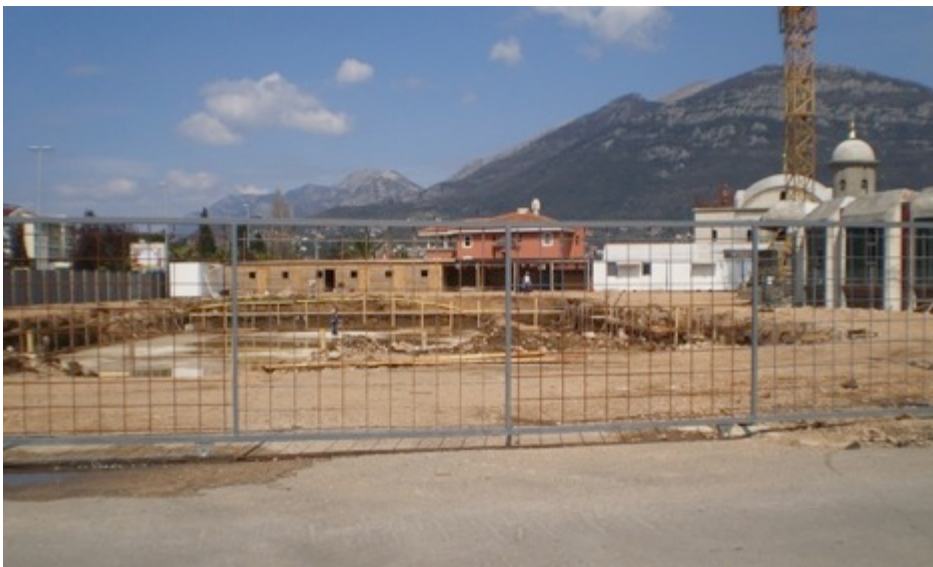
Figure 15: The construction site of an allegedly illegal construction in the centre of Bar, May 2011 (Photo: MANS (UNFPA 2007)).
