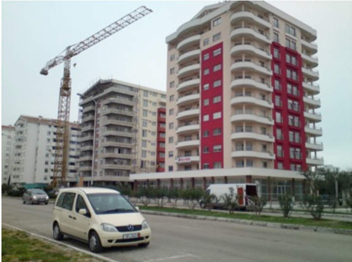
On-going construction of apartment buildings in the centre of Bar, an urbanized area.
